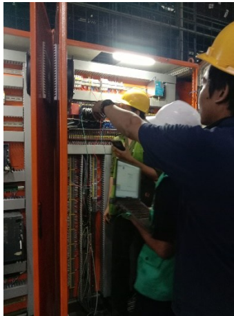
Gambar 4. 23 Proses commisioning program pada panel control PT. Elang Perdana
