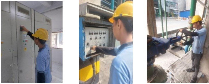
Gambar 4. 18 Start or Stop Pompa Cooling Water
