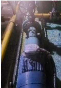
Gambar 3. 12 DC Emergency Oil Pump
