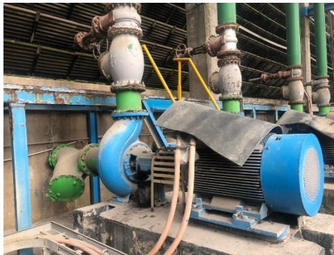
Gambar 3. 26 Pompa Sirkulasi Cooling Tower
