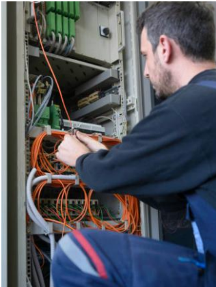
Gambar 3. 2 Pengecekan kabel Patch Core
