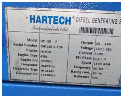
Gambar 2. 12 Nameplate Generator Set Hartech 25 F
